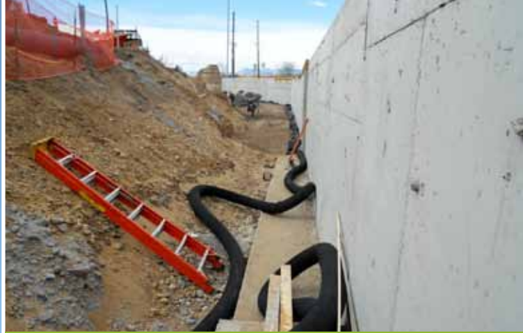
Drainage system ready for installation behind the retaining wall at Washington Street and 68th Avenue. (Photo courtesy of Adams County.)
