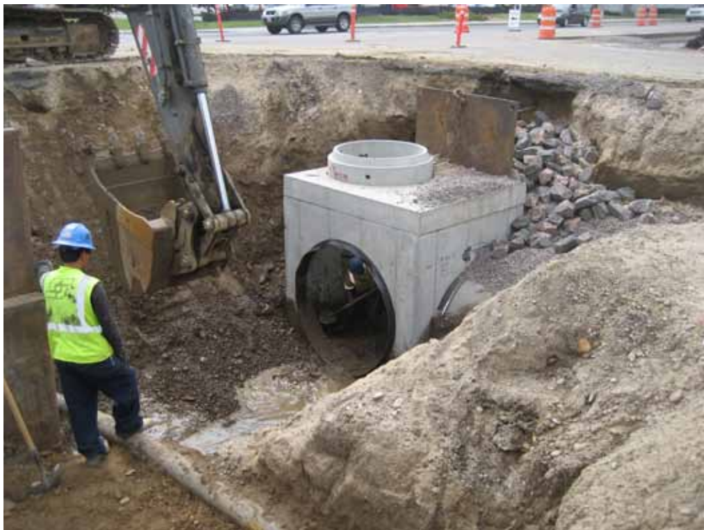
A box base manhole is installed. (Photo courtesy of Scott Contracting Inc.)
