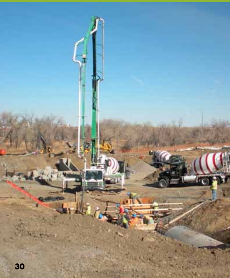
Pumper truck onsite to pour overflow structure on toe walls for outfall structure. (Photo courtesy of Adams County.)
