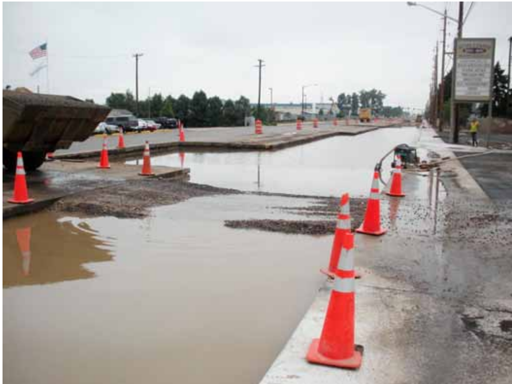
A major rainfall left pools that had to be pumped out prior to resuming construction. (Photo courtesy of Scott Contracting Inc.)
